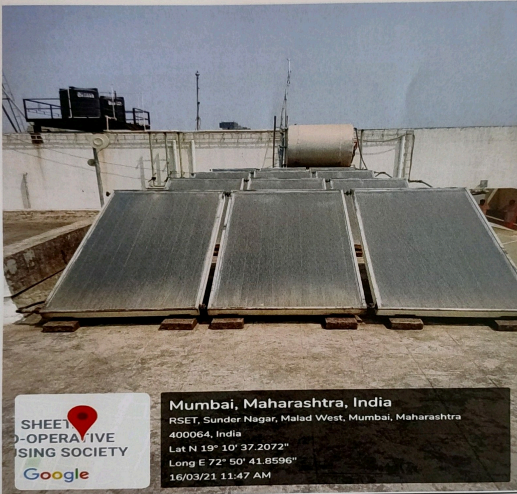
Solar Panels for energy conservation in the campus
