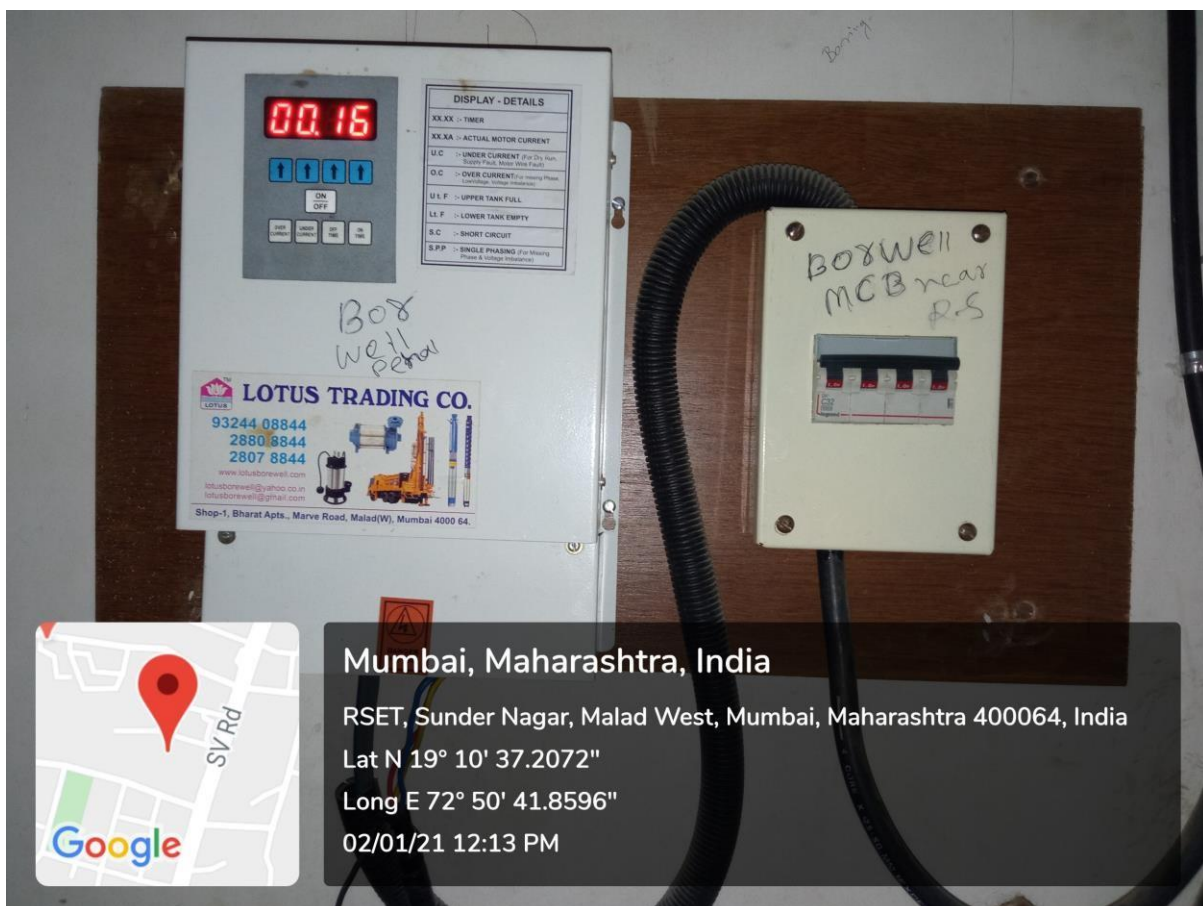
Bore well Panel
